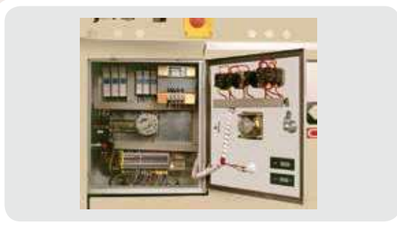
Electrical box with safety and integrated controls
